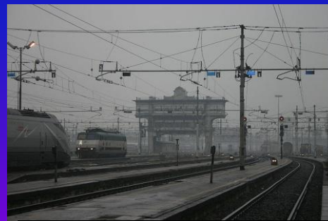
Railway data communications
