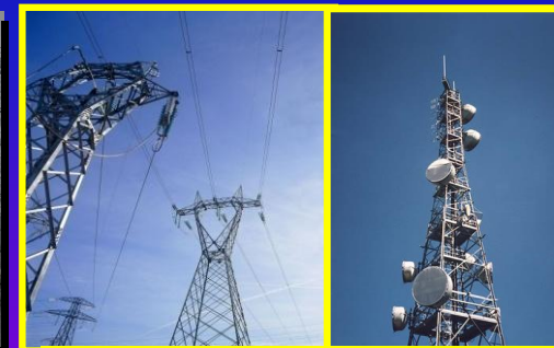
Electric Energy . Data & Speech Transport (PLC)
